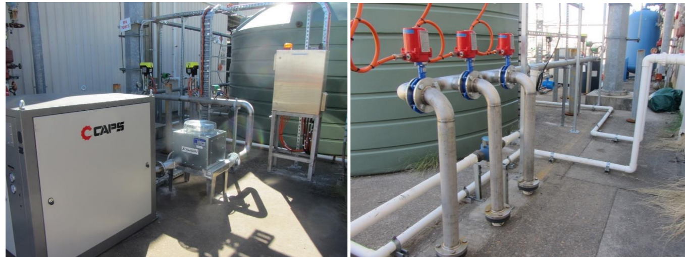
Photo 1: Blower, cooler, control cabinet and piping.
